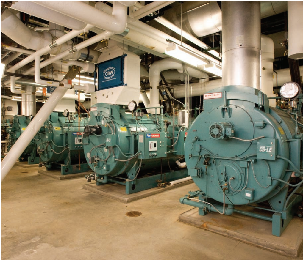
Gundersen Lutheran Health System changed the way their boilers were being used. Converting high-pressure steam to low-pressure allows them to turn off several boilers in one of their outpatient buildings, saving the health system nearly $64,000 annually.
